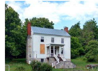
South Side restored. Now rear entrance. Plywood covers kitchen window under restoration
